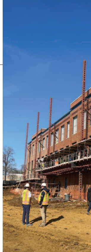
In November 2021, demolition of the greenhouse keepers quarters began alongside College Creek. Construction of the Fluegel Alumni Center began in early 2022. The new facility is scheduled to be complete by June.
