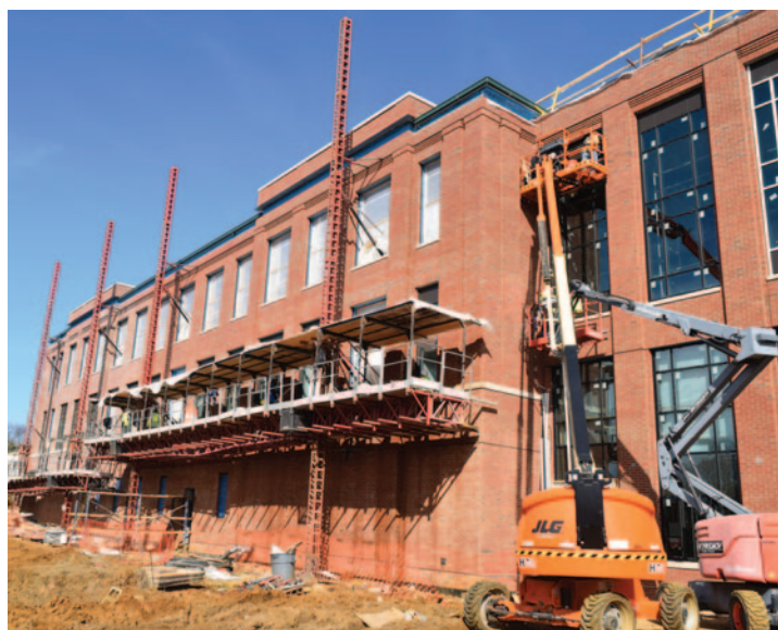
Construction of the Fluegel Alumni Center continued during February. The 65,000-square-foot facility is scheduled to be complete in June. A legacy gift from Donna and Rick Fluegel '61 helped ensure the Naval Academy alumni community has a first-class home in Annapolis.
