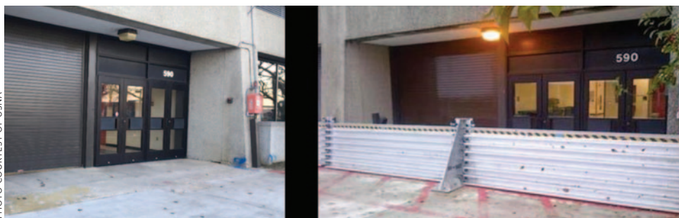
Door dams are utilized outside Rickover Hall to protect the low-lying entrance.
