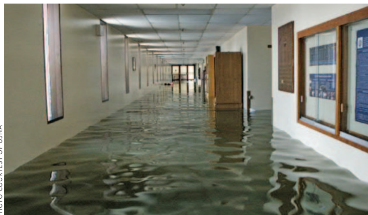
Chauvenet Hall’s Laboratory Deck was flooded during Hurricane Isabel. That storm caused nearly $100 million in damages to the Yard.
